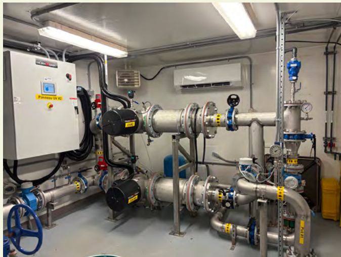
Station Riverview qui alimente le village
